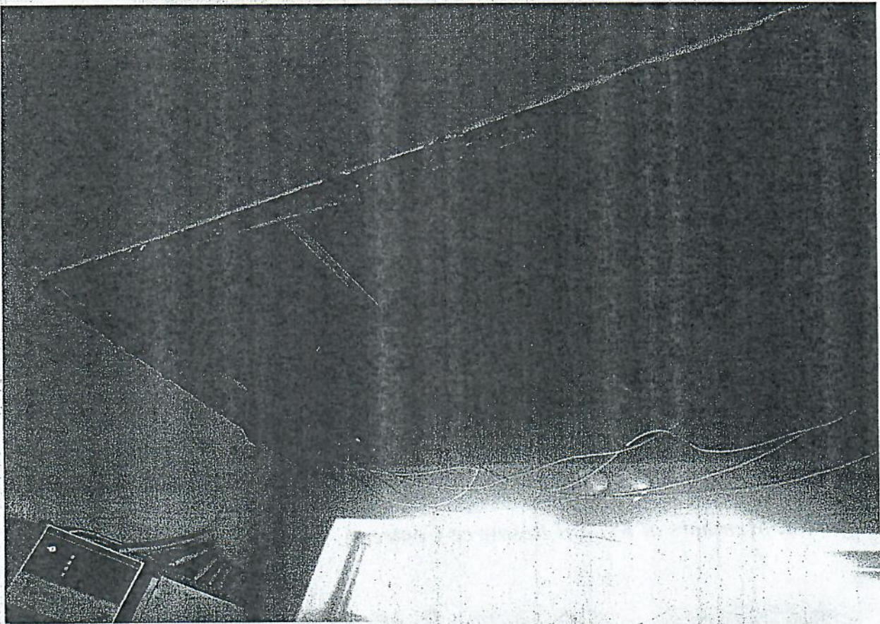
Figure 7. A portion of ceiling that has fallen off at the Kyoani Resource Centre.
