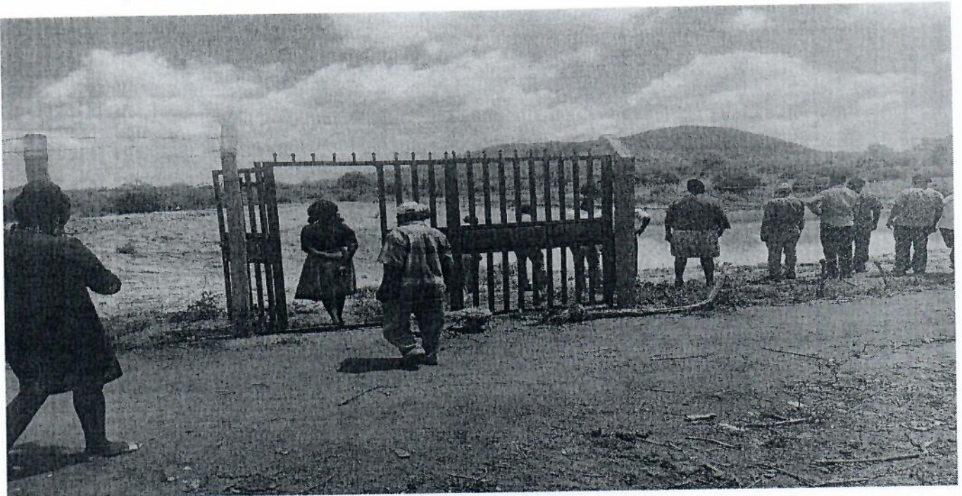
The gate at Kitambasye earth dam that is loosely tied with binding wires.
